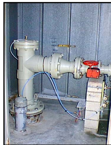
Seawater Barrier Injection Well
